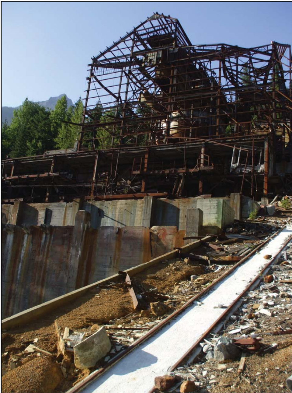
Figure 5.8: The skeleton of an old mill building at the Holden Mine site.
