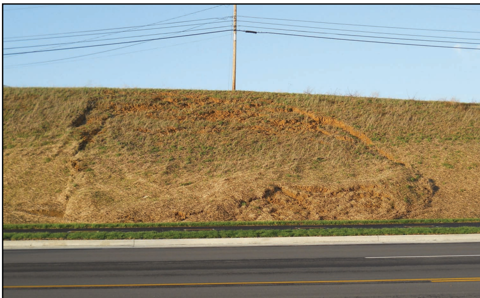
Figure 9.14: A small slump in a road embankment along KY-421 in Franklin County, Kentucky.
