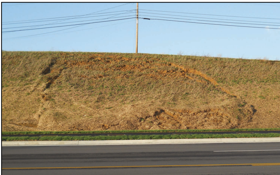
Figure 9.14: A small slump in a road embankment along KY-421 in Franklin County, Kentucky.
