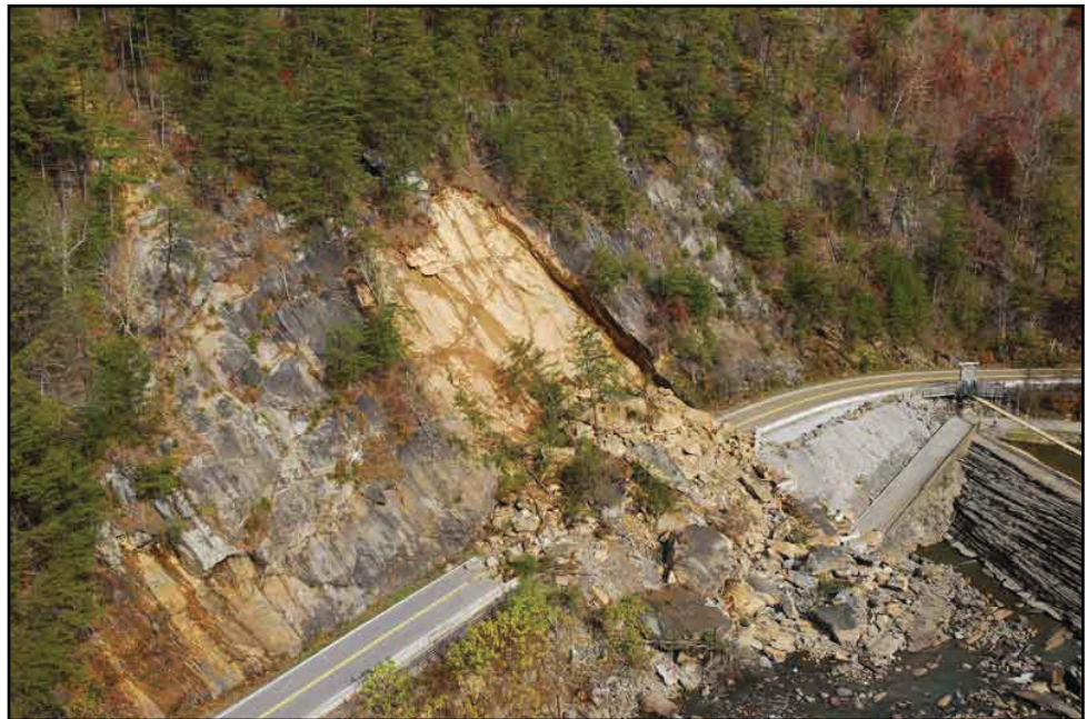
Figure 9.11: This rockslide across US 64 in Polk County, Tennessee, resulted in an eight-week-long road closure while the rocks were removed.
