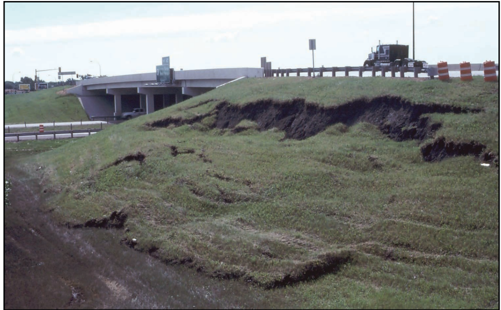
Figure 10.16: This slump near Interstate 29 in Fargo, North Dakota occurred in clay-rich materials used to construct the nearby overpass.
