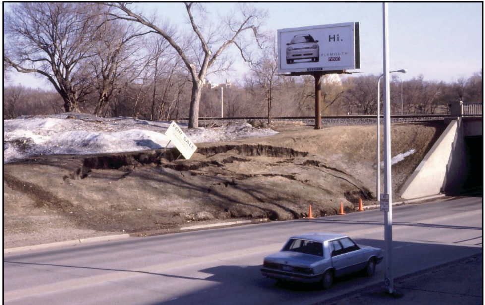
Figure 10.17: This slump occurred along a North Dakota roadcut after a spring thaw melted piles of snow on the upper bank, saturating the clay-rich soil and increasing its weight.
