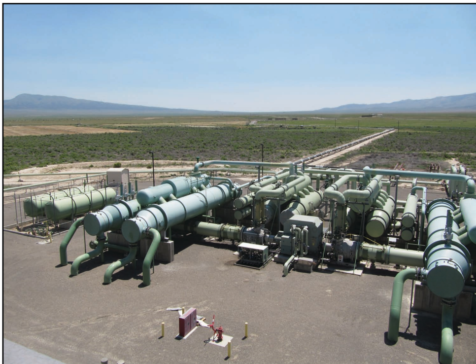
Figure 7.17: The 13 MW Raft River Geothermal Plant near Malta, Idaho was the first commercial-sized binary cycle geothermal plant in the world. The plant's condensers and heat exchangers are pictured here.
