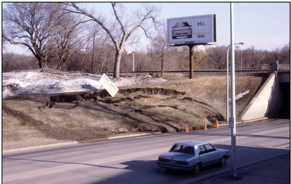
Figure 10.17: This slump occurred along a North Dakota roadcut after a spring thaw melted piles of snow on the upper bank, saturating the clay-rich soil and increasing its weight.
