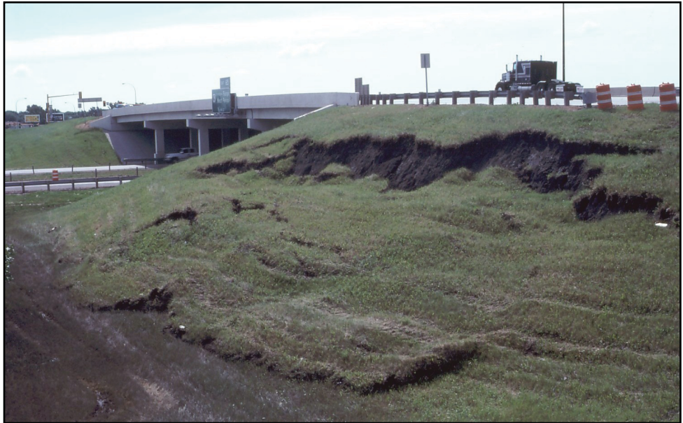
Figure 10.16: This slump near Interstate 29 in Fargo, North Dakota occurred in clay-rich materials used to construct the nearby overpass.
